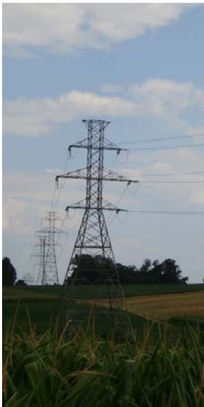
Figure 4.8 - Expansion of existing transmission lines is a threat to the scenic quality of the Byway and must be monitored very closely
