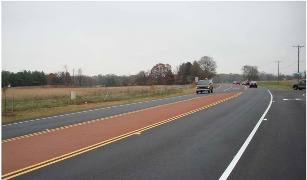
Figure 4.33 - Example of tinted asphalt used to break up the wide visual expanse of pavement - along with rusting steel guardrails. - construction photo for Route 15 in Virginia
